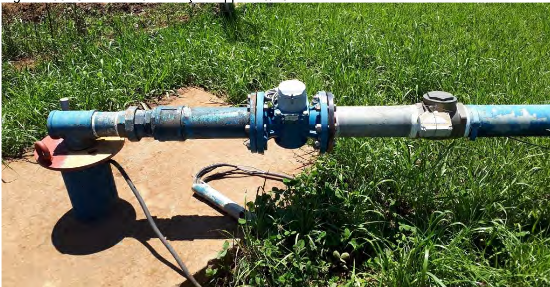
Figura 109: Cavalete P07 – Poço Tieppo -10/2022.
