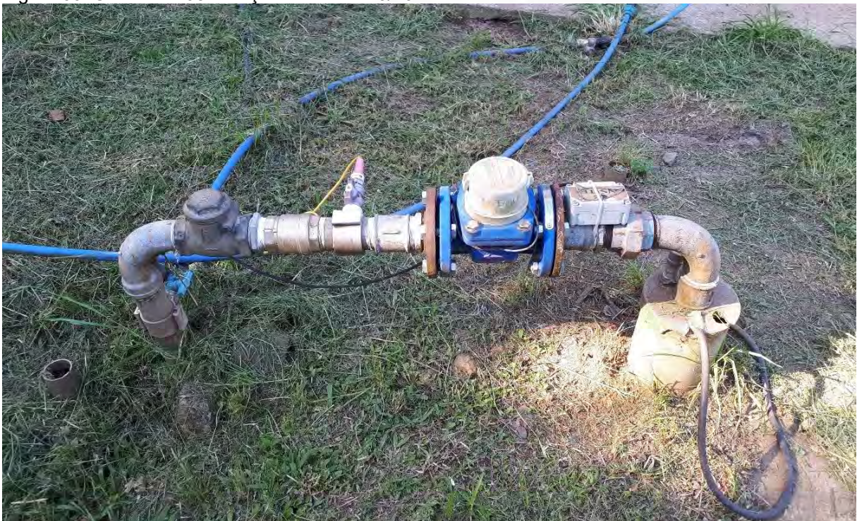
Figura 66: Cavalete P08 – Poço Vila Nova -10/2022.
